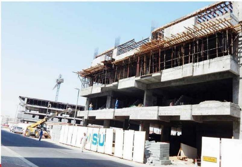
Project: 2B+G+9+R Comm.office/Resi. Building Location: Plot No.246-170 @ Al Qusais Ind.3 rd Client: Abdalkarim Abdulmajeed Shahada Abudaqqa
